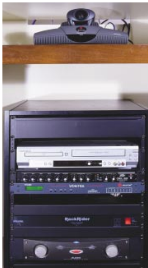
A streamlined rack of source equipment is easily accessible at the front of the room.
